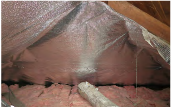
Radiant barrier installation is a simple, effective treatment for homes in hot climates.
